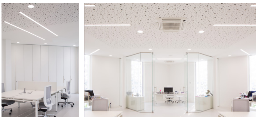
Linear luminaires combined with point light sources are discreetly integrated into the ceilings of the office area.
